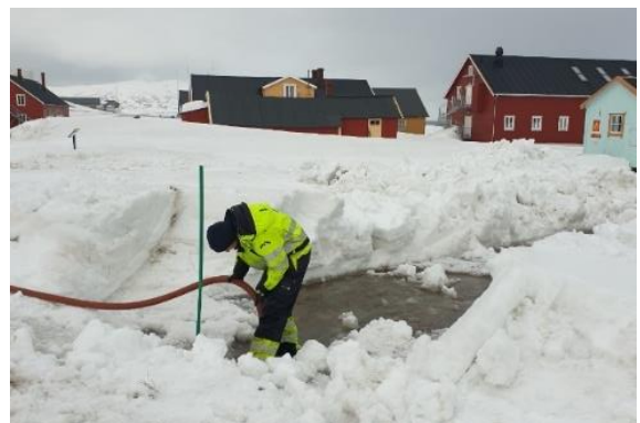
Figure 12. Clogged culverts, March 2022
