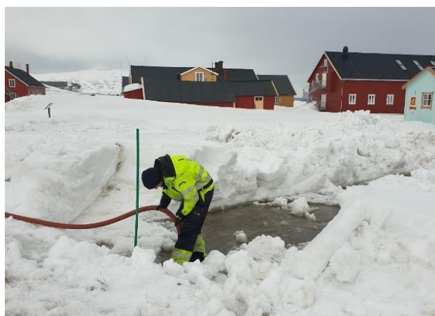
Figure 13. Clogged culverts, March 2022
