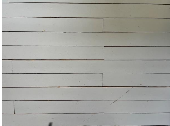
Malt bordgulv, sprekker grunnet krymp.
