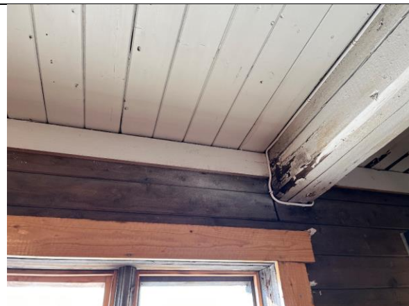
Opprinnelig/eldre malt faspanel i himling.
